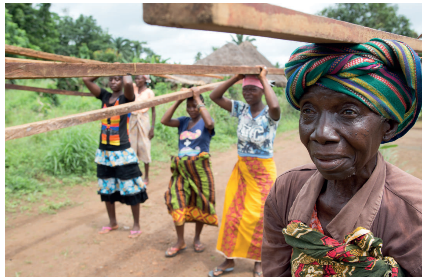
Women building a new health clinic in the village of Sawula, in the Pujehun district of Sierra Leone. Picture credit: Christian Aid / Tom Pilston
